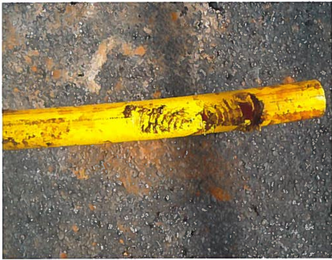
Natural gas piping damaged during cleanout operations
