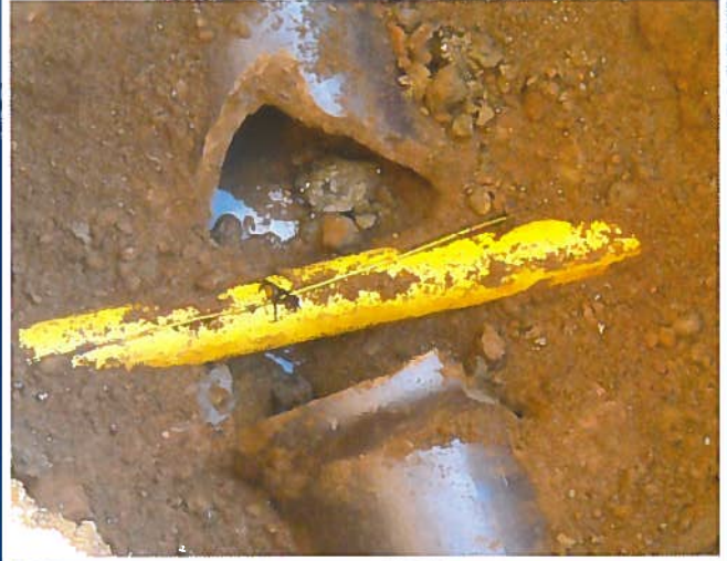
A sewer line penetrated by natural gas piping
